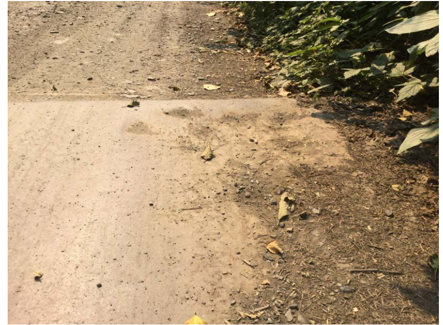
Steel deck plate deformation, up to 25mm deformation in locations
